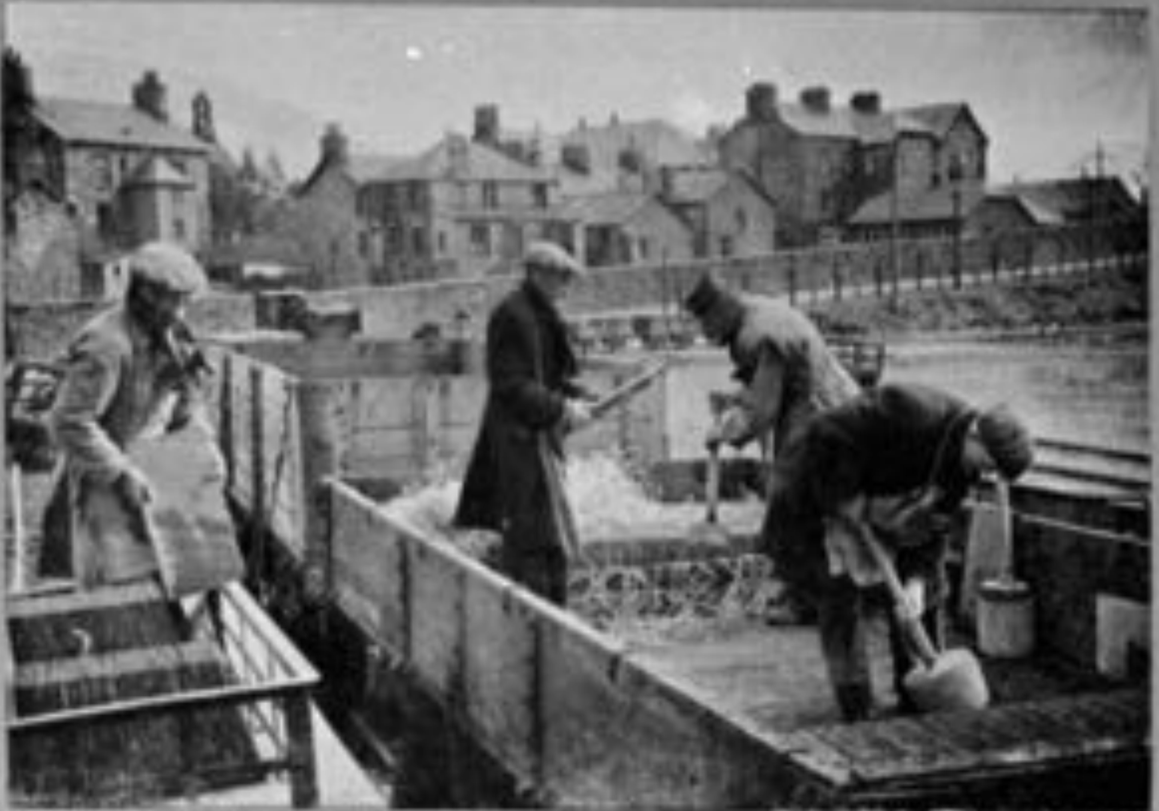
(Above) Using the "matless" in a low-sided railway wagon. It is better in the long run to handle only a few slates at a time.
