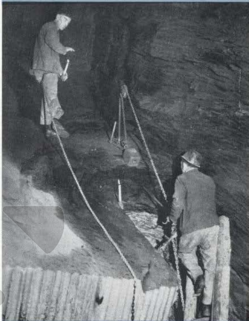
(Above.) The first task is to free the great slab. The rock having already been cut across with a channelling machine, the rockmen are now cutting a "free side."
