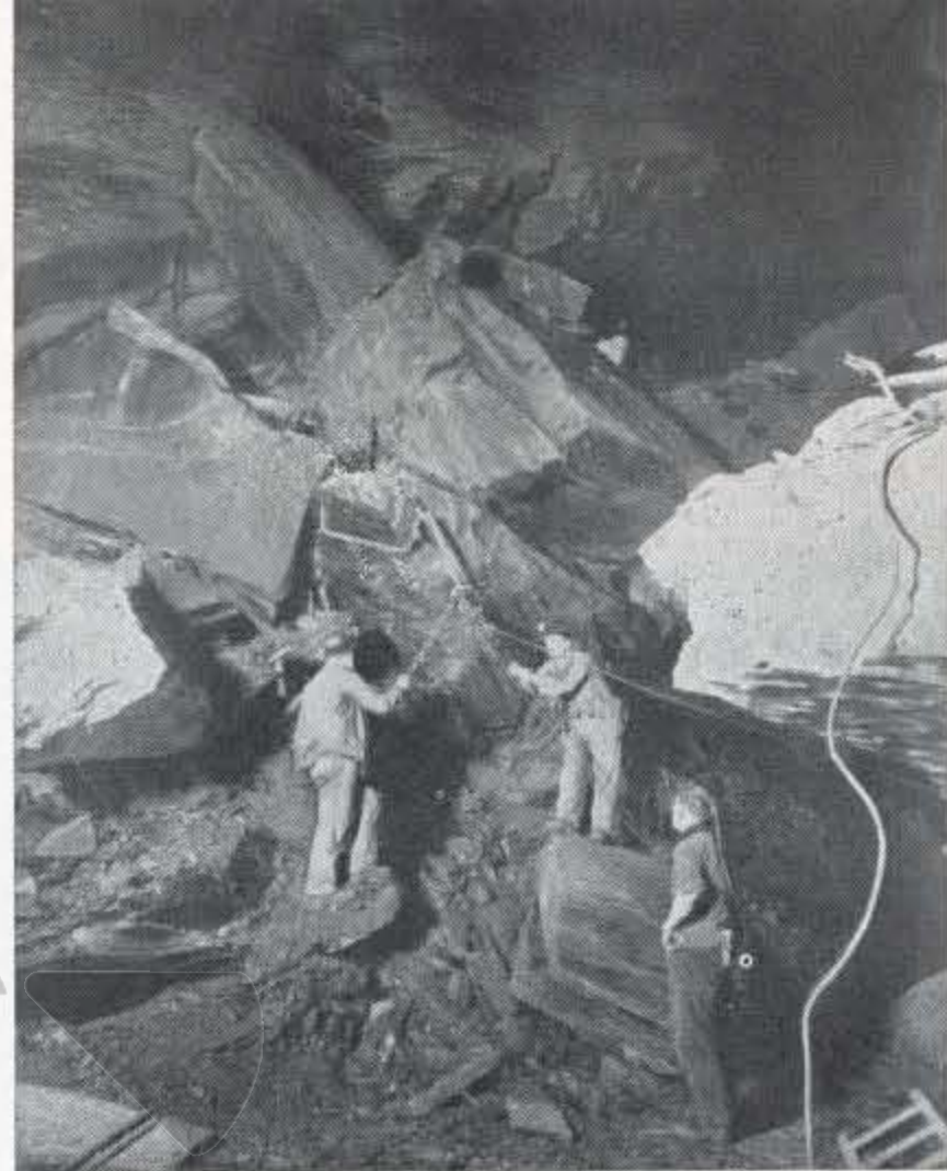
Preparing to extract a block from the rock-fall, a task made easier with air-winch and stout wire ropes.
