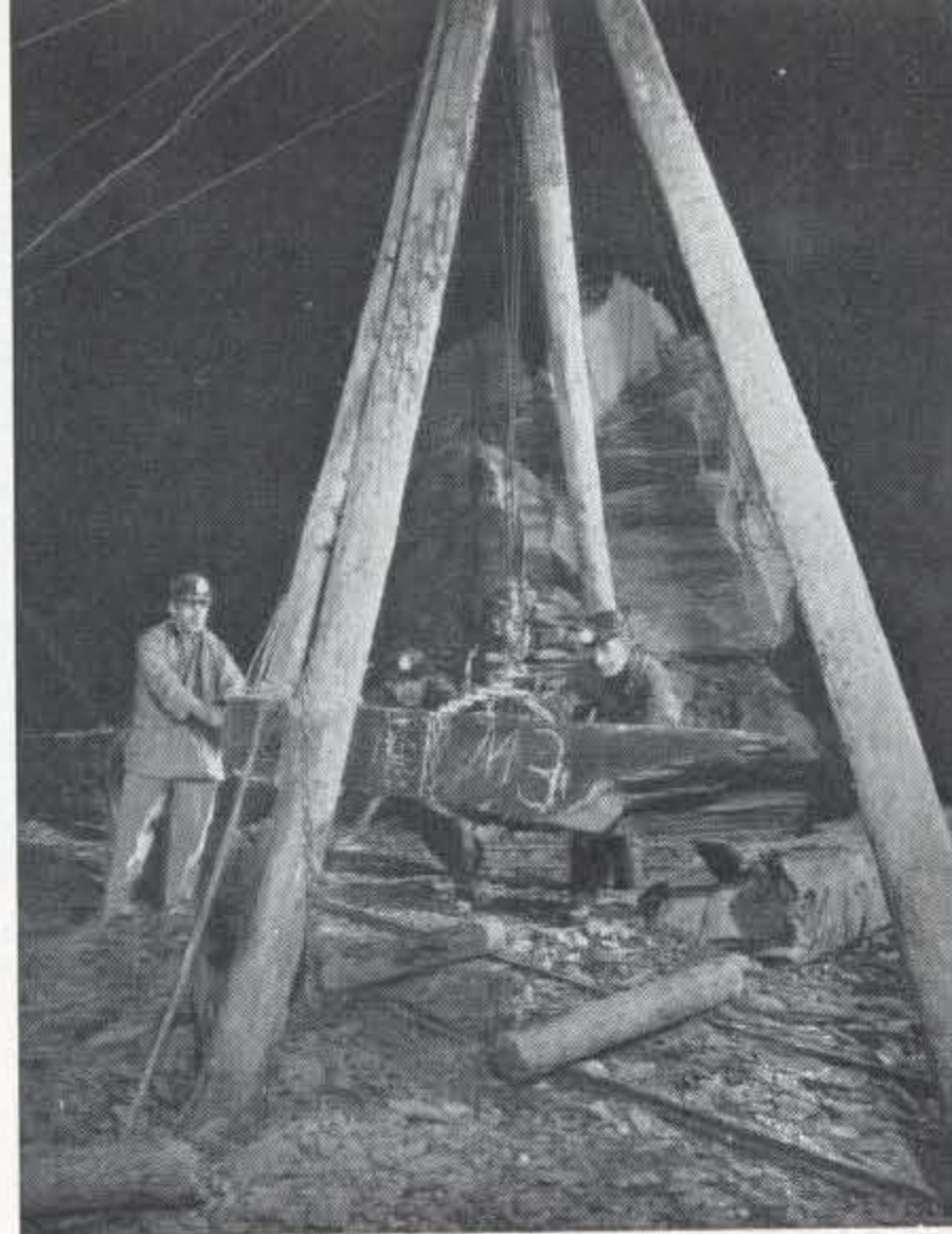
A block of manageable size, now identified by the partnership symbol M3, is hoisted by air-winch for loading on to a trolley to be run underneath.
