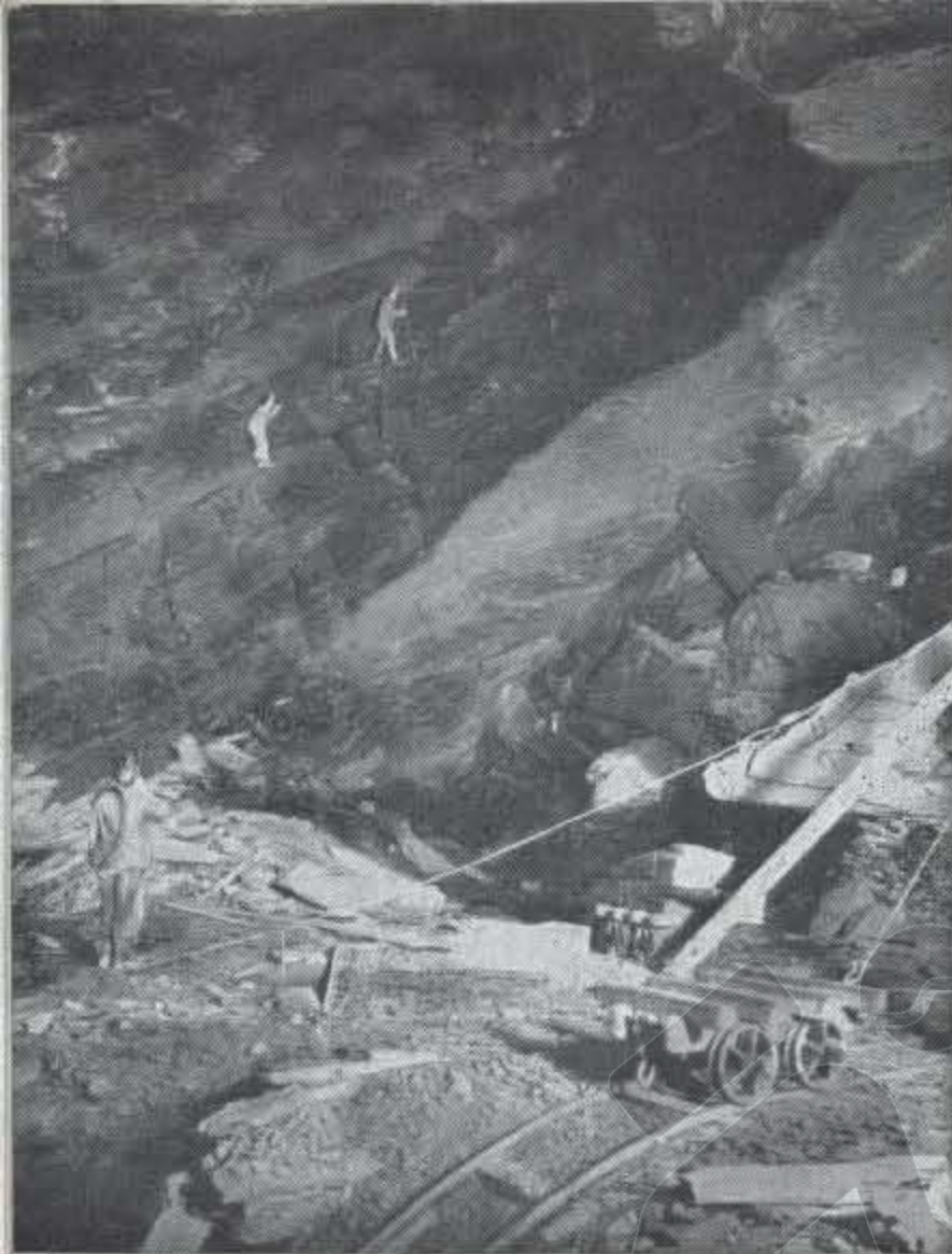
Core of the mountain—the slate in situ. Rockmen get to grips with the slate in the mass. The scene of operations is the "high level" section of M3.
