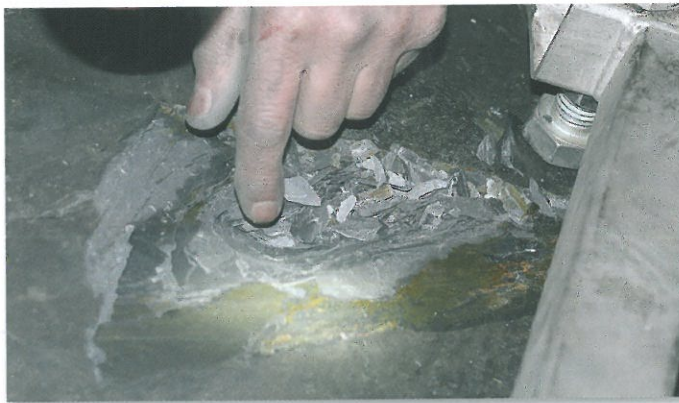
Typical spalling of surface layers following extraction of an anchor
